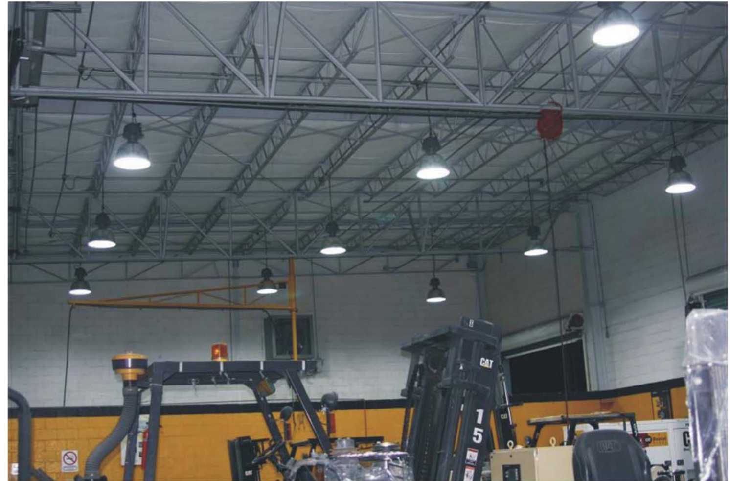
SP-7006, Caterpillar Service Center, Mexico 73
